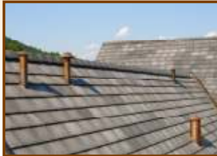
Copper Roof Vent Sleeves
